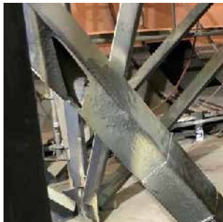
Eroded Structural Members
