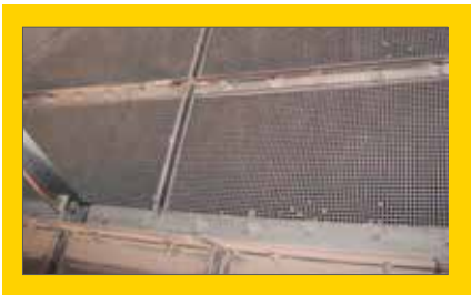
Conforma Clad screens after nine months.
