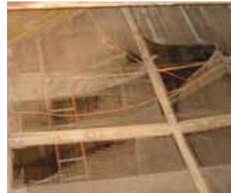
Stainless steel screens after less than six months performance.
