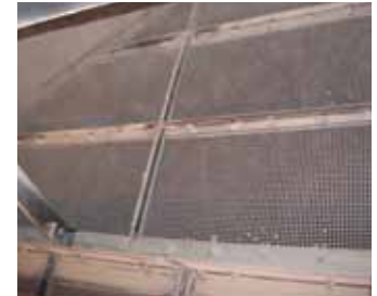
Kennametal Conforma Clad screens after nine months.
